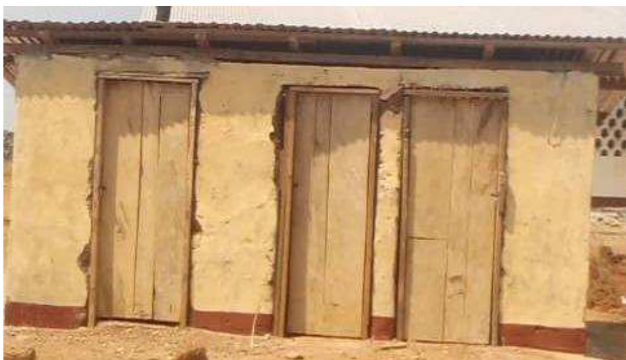
3-compartment toilet handed to EP Mayo - Linwa
