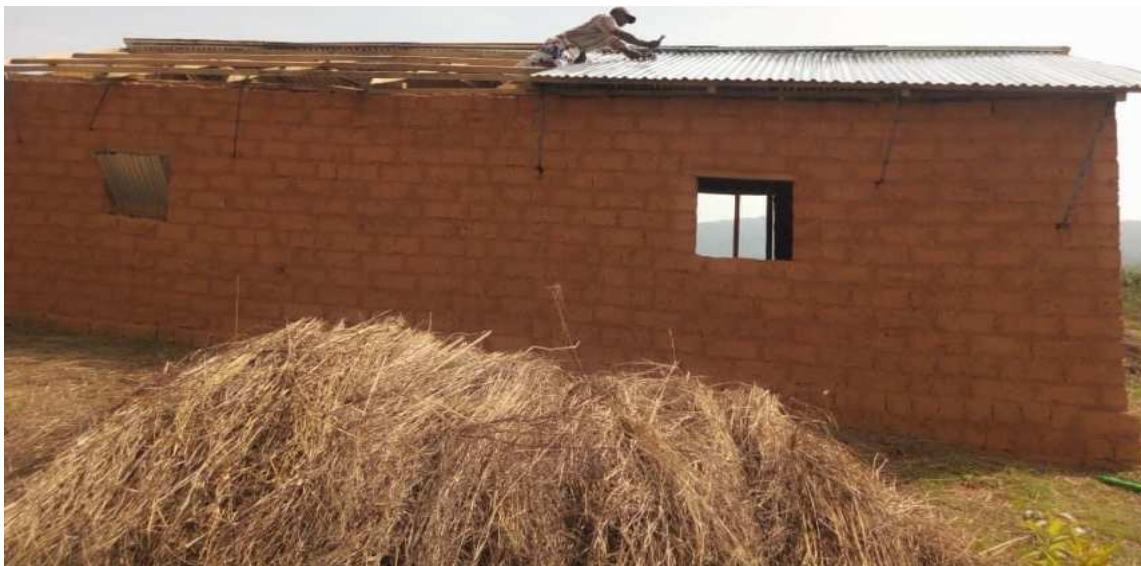
Classroom destroyed by wind
