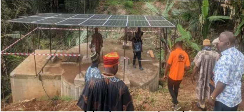
Solar that powers the tank
