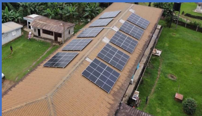
120 Solar panels mounted on the roof of the building
