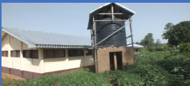
Installed water tank at GBHS
