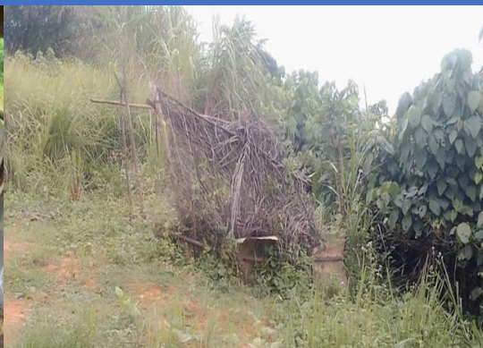
Toilet in a dilapidating state
