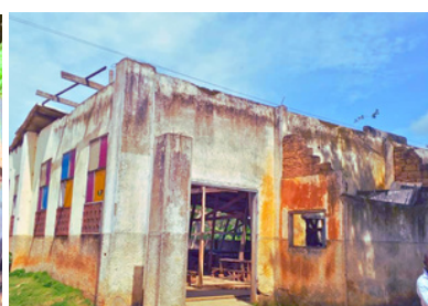
Some Pupils using this dilapidated building before
